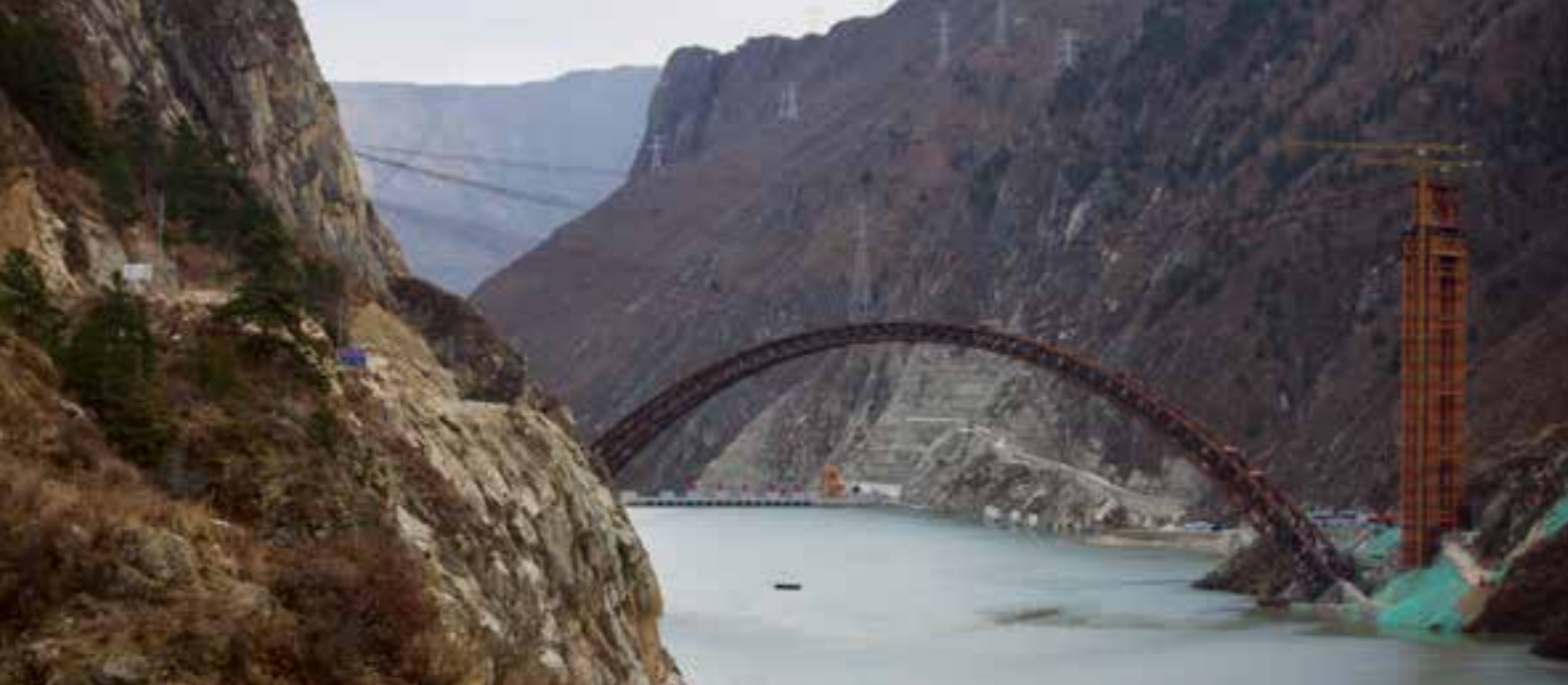
The Lhasa-Chengdu Railway is being built through the mountainous Tibetan region. In this photograph, the construction crosses in front of the Zangmu Hydroelectrical Dam.
